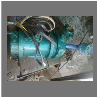
Water Pump Motor
