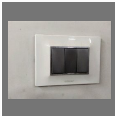
Electro Switch Board
