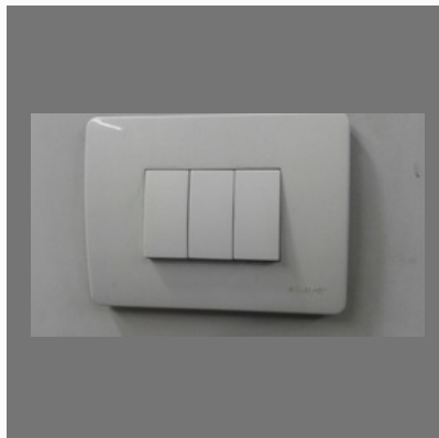
White Switch Board
