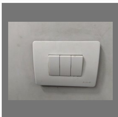
White Switch Board
