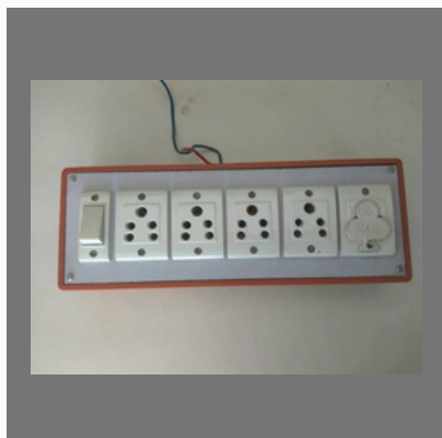
Electric Switch Board
