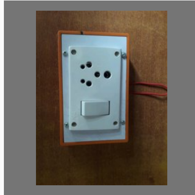
Electrical Switch Board
