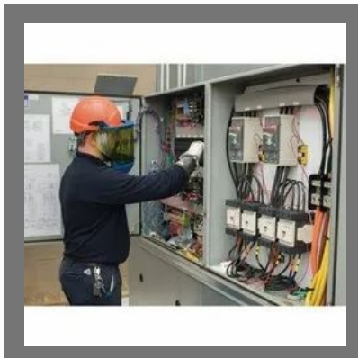
Industrial Electrical Service
