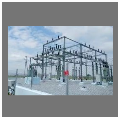
Electrical Turnkey Project
