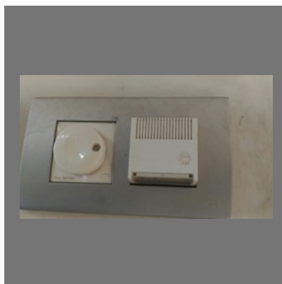
Fan Regulators Switching Device
