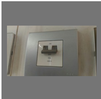
High Voltage Switch
