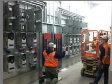
Industrial Electrical Installation Services
