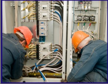
Electrical Installation Services
