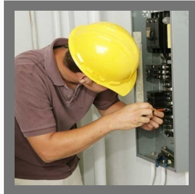
Residential Electrical Contractor
