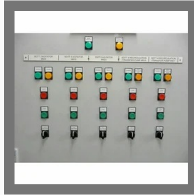
Industrial PLC Control Panel
