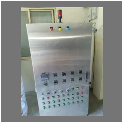
MCB Control Panel
