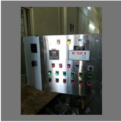
Automation Control Panel
