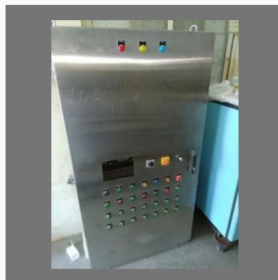
Siemens Control Panel
