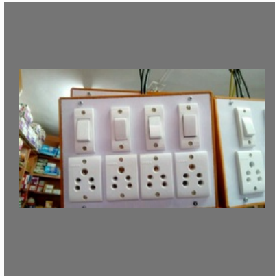
Electrical Switch Board
