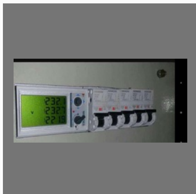
MCB Distribution Boards
