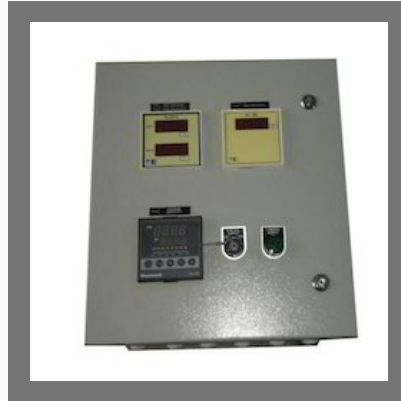
Control Panel Board
