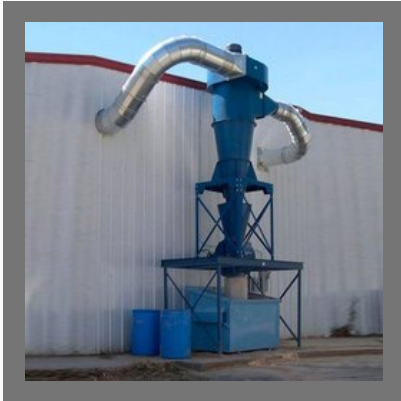
Cyclones Dust Collector
