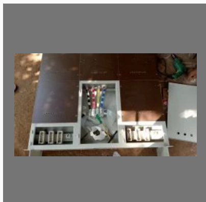
Electrical Control Panel Board
