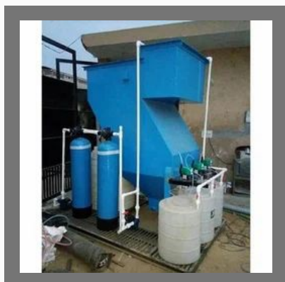
Effluent Treatment System
