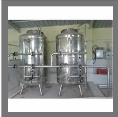
Softener Water Treatment Plant
