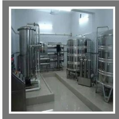
Automatic Softener Water Treatment Plant
