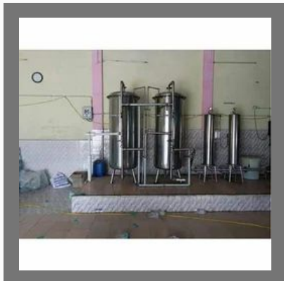
Automatic Industrial RO Plant
