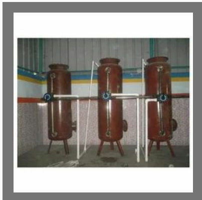
Vertical Water Treatment Plant
