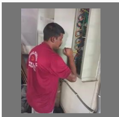
Inverter Wiring Service
