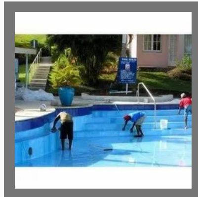
Swimming Pool Plumbing Service
