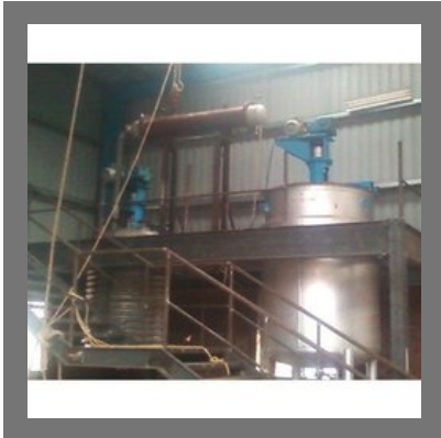
Ploythethane Resin Plant
