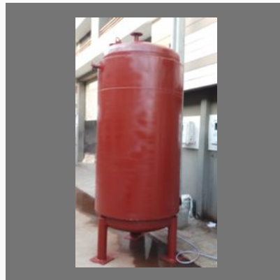
MSRL Storage Tank
