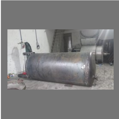
FO STORAGE TANK
