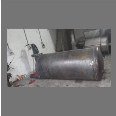
MSRL DM Plant Tank
