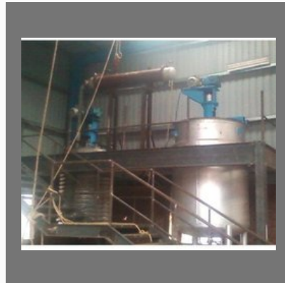
UNSATURATED POLYESTER RESIN PLANT
