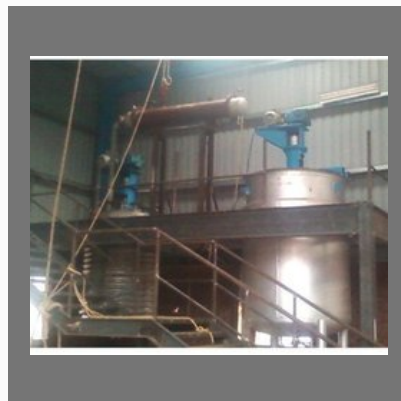
UNSATURATED POLYESTER RESIN PLANT
