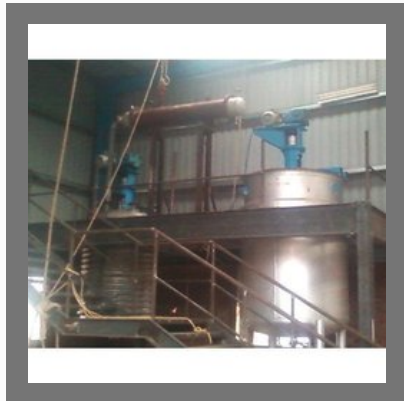
Ploythethane Resin Plant
