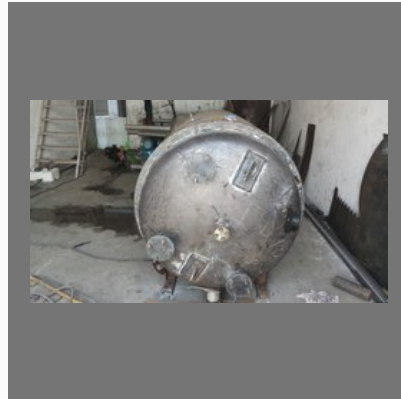
FUEL STORAGE TANK
