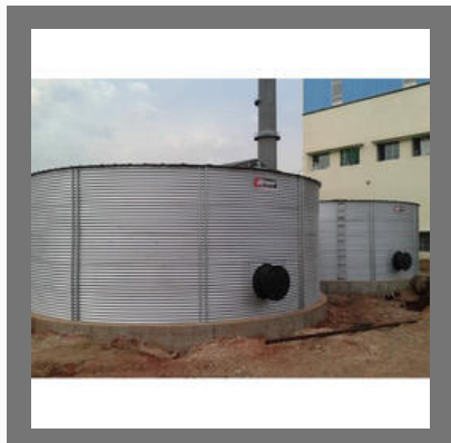
Effluent Water Tank
