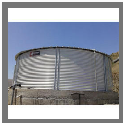
Diesel Oil Storage Tank
