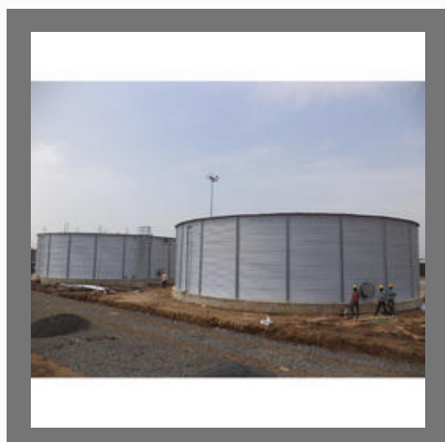
Fire Hydrant Tank
