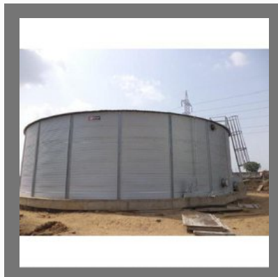
Chemical Storage Tank
