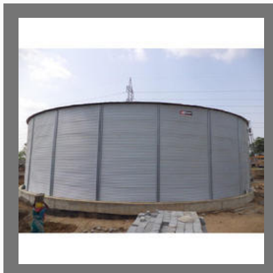
Oil Storage Tanks
