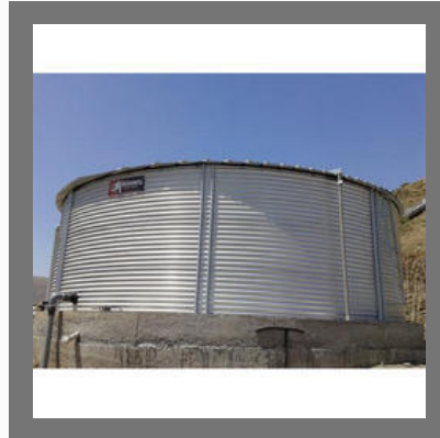
Raw Water Tank
