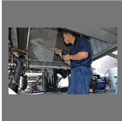
AHU Duct Cleaning Service
