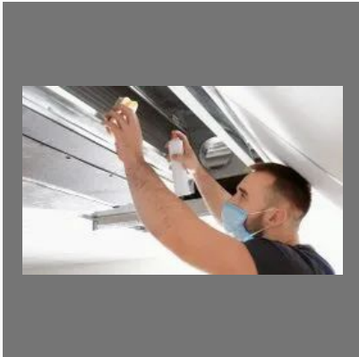
Hospital Duct Cleaning Services
