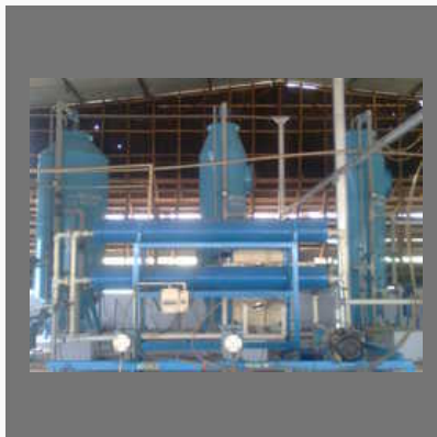
Waste Water Treatment
