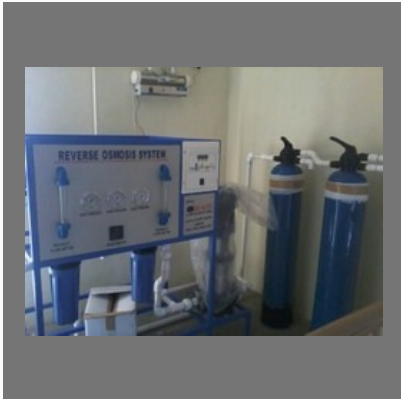
Sand Filter Carbon Filter U.V
