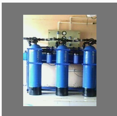
Sand Filter Carbon Filter With Softner
