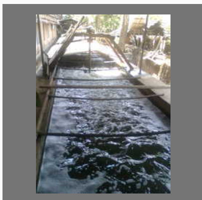
Sewage Treatment Plant Hospital Waste Water
