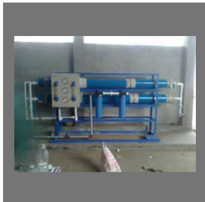
Waste Water Treatment
