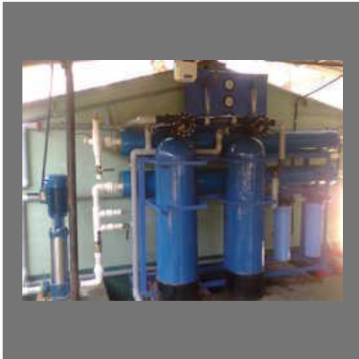
Sewage Treatment-R.O. System
