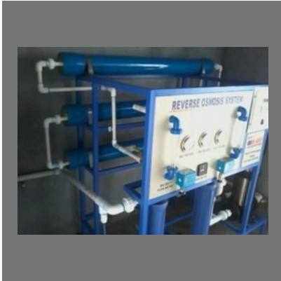
Sand Filter Carbon Filter Automatic
