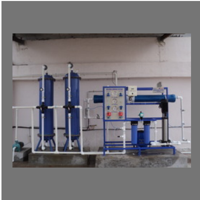
Ms Sand Filter Carbon Filter Automatic
