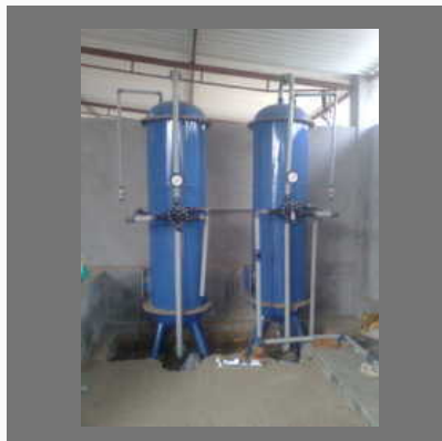
Sand Filter Activated Carbon Filter Municipal Water
