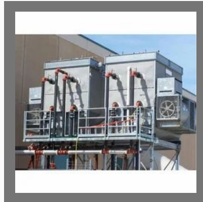
Commercial Rooftop Air Conditioning Unit
