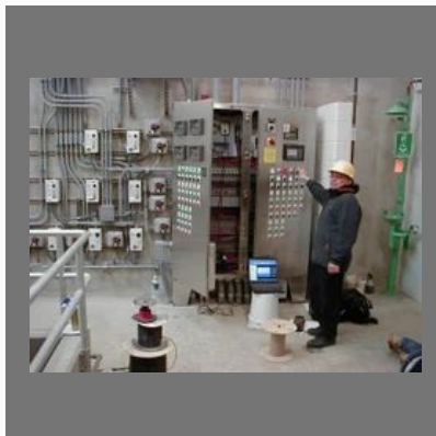
Electric Control Panel Installation Service
