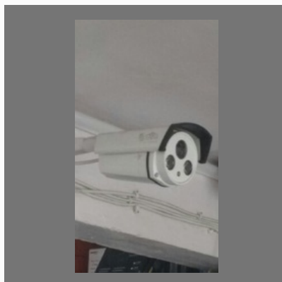
HD CCTV Camera
