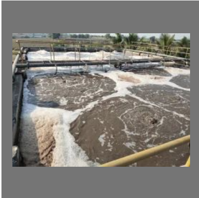
Sewage Water Treatment Plant Service
