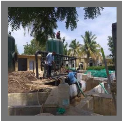
Waste water Treatment Plants Service
