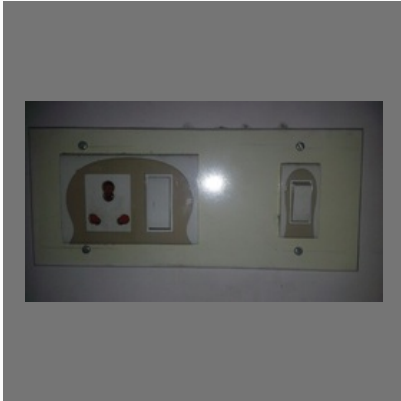
Modern Switch Board
