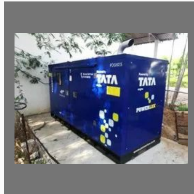
TATA Motor Diesel Generator
