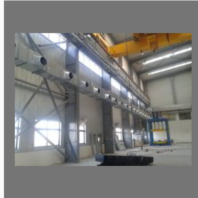
Air Washer Supply Duct
