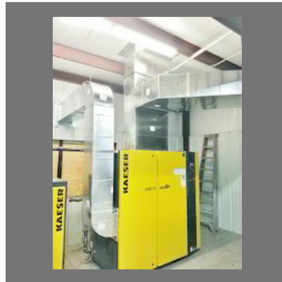
Compressor Air Duct
