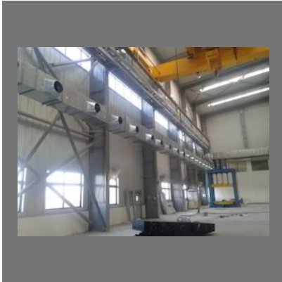
Air Washer Cooling Duct
