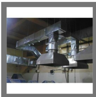
Hot Air Exhaust System
