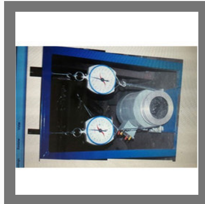
Synchronization Control Panel
