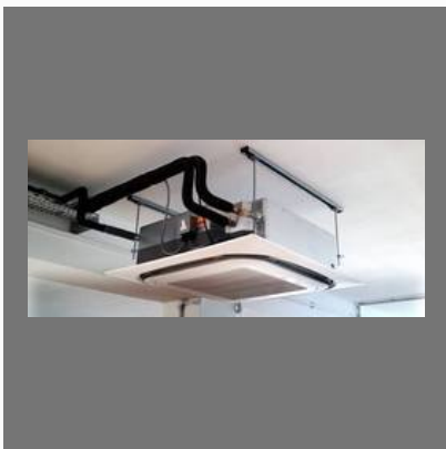
AC Cooling Systems
