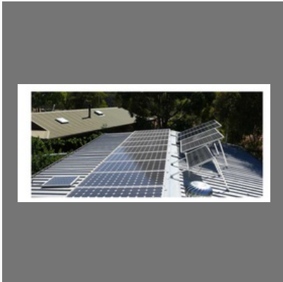
Solar Home System
