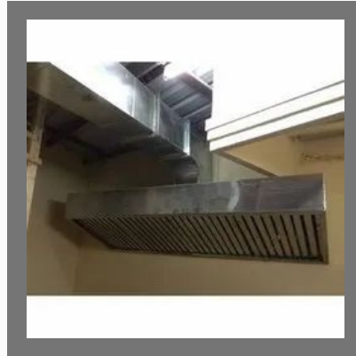
Commercial Kitchen Hood
