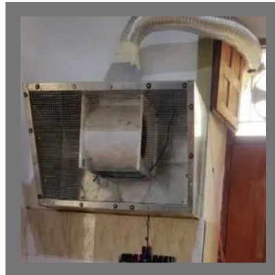
Commercial Kitchen Chimney
