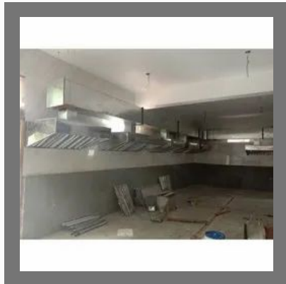
Industrial Kitchen Chimney
