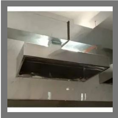
Kitchen Exhaust Hood
