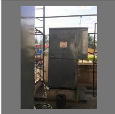
Electrical Inspection Compliance Reports
