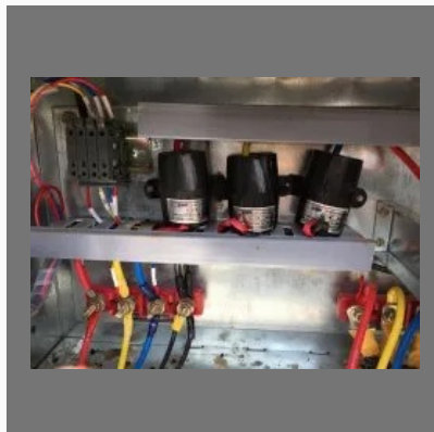
Electrical Earthing Testing
