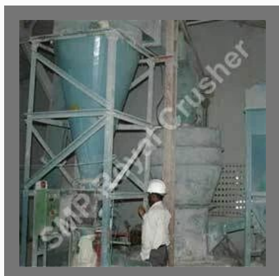
3 Roller Grinding Mill
