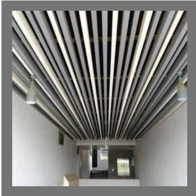
False Ceiling Services
