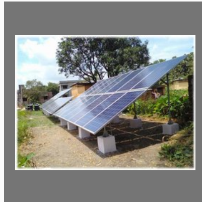
Ground Mount On Grid Solar System
