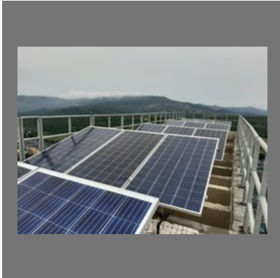
On Grid Rooftop Solar Panel System
