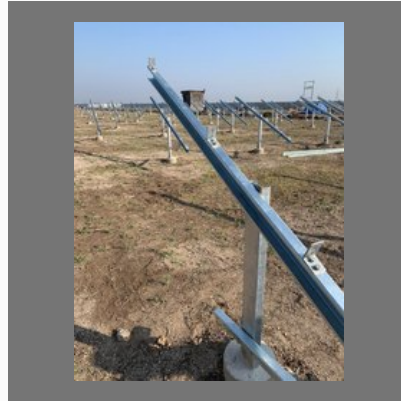
Solar Panel Mounting Structure
