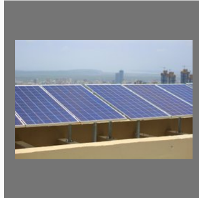
On Grid Solar Power Systems
