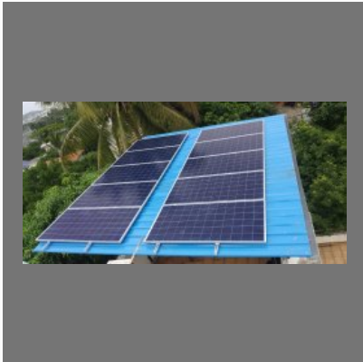
Residential Solar Rooftop System
