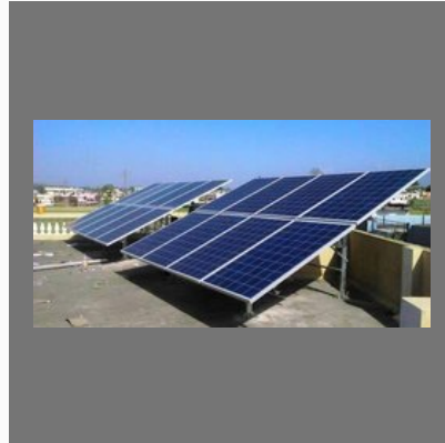
Residential Solar Rooftop System
