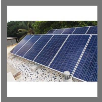
Solar PV Power Panel
