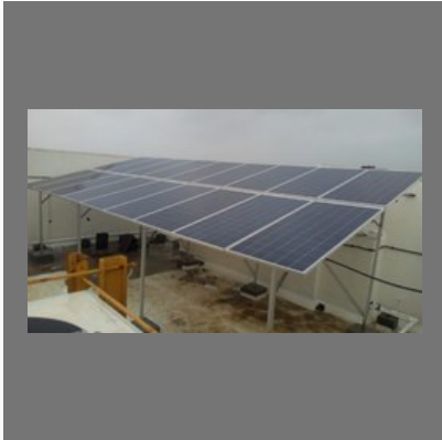
6kWp On Grid Solar System
