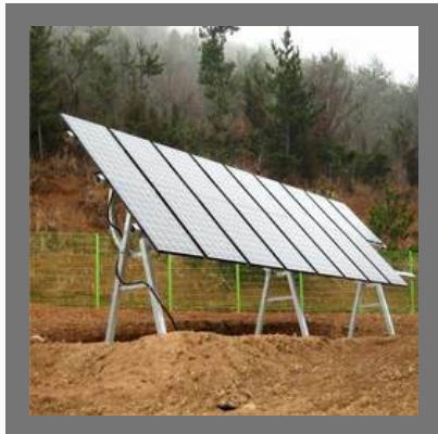
Solar Power Plants
