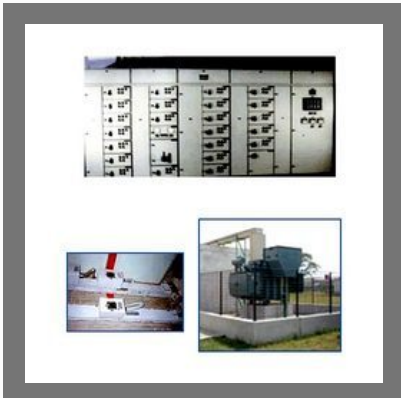
Bus Duct & Main Panel
