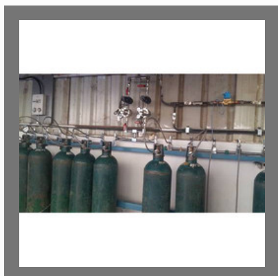
Medical Gas Pipeline
