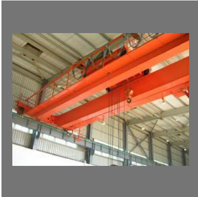
Eot Crane Over Head Crane
