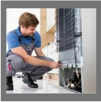
Refrigerator Repair Services
