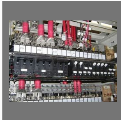
Electrical Installation Services
