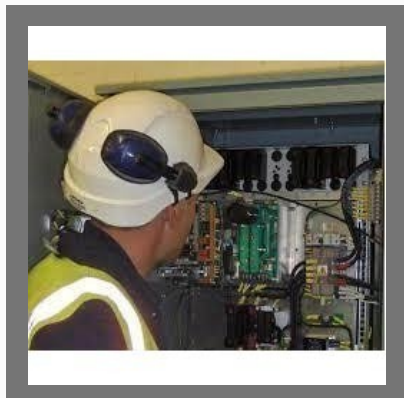
Electric Commissioning Services
