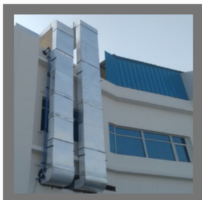
GI Ducting / Ducting
