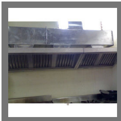
Cooking Area Ventilation System
