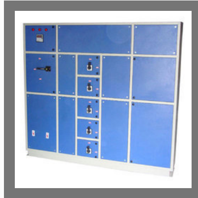
Sub Switch Box
