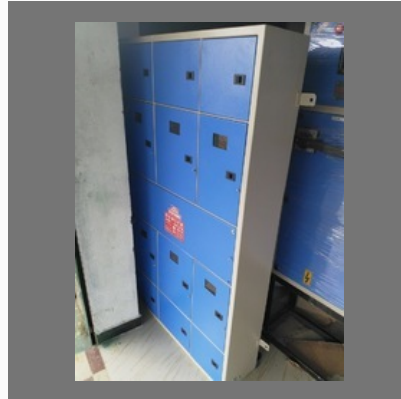
Multiple Metering Panel
