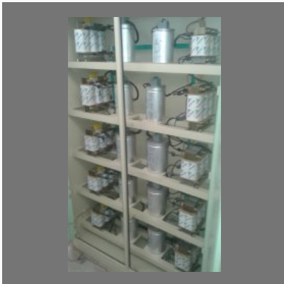
Automatic Power Factor Control Panel
