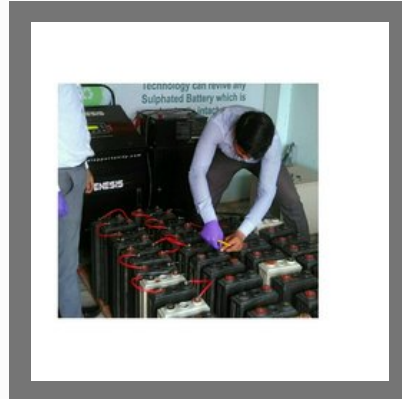
Battery Health Checkup
