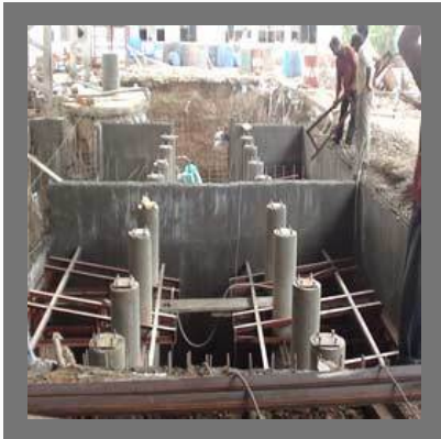
Heavy Duty Paint Booth Machine Foundation
