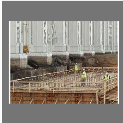
Machines Foundation Services
