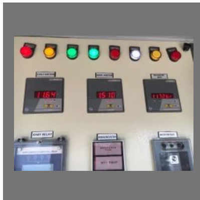
Industrial Electrical Services
