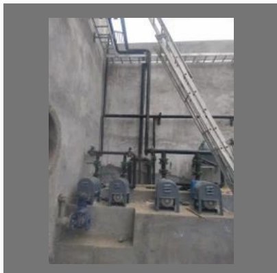
Mechanical Contractors Service
