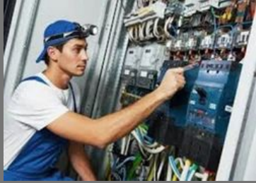
Facility Management Services
