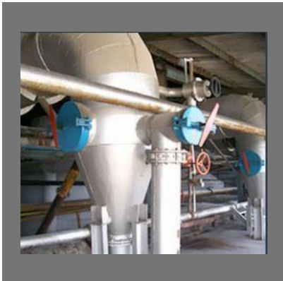
Cooling And Condensing Systems
