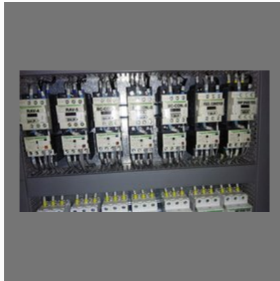
Feed Conveyor Control Panel
