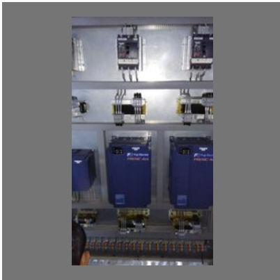
ACE Control Panel
