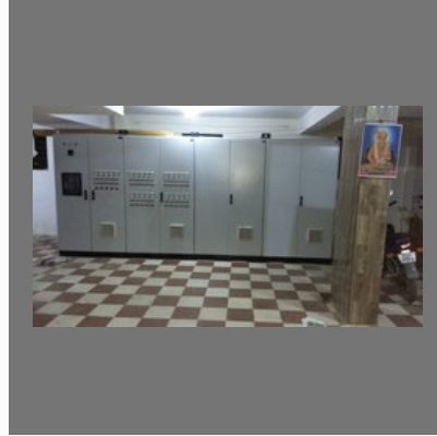
Motor Control Panel Board
