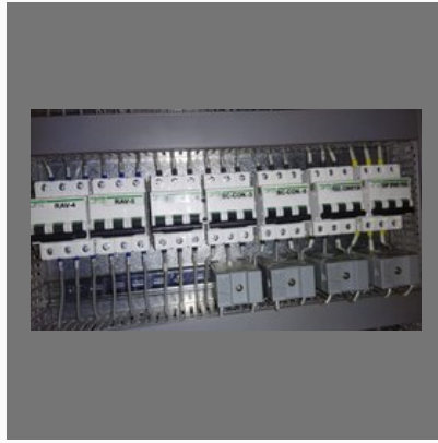
BC Conveyor Control Panel
