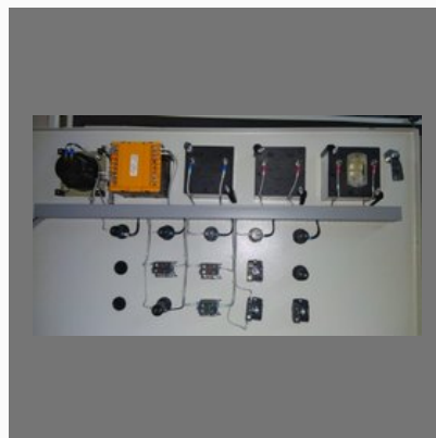
PLC Control Panel Board
