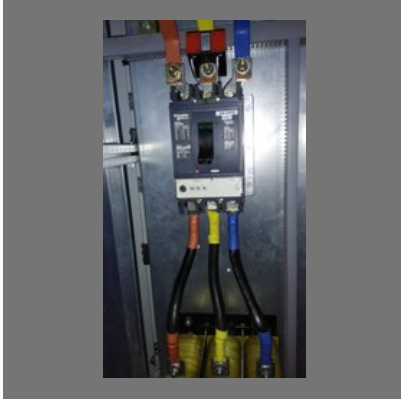
Single Phase Control Panel Board
